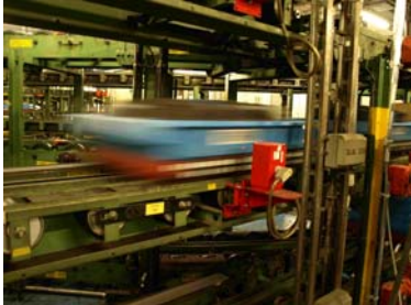
P3313095, P3313096: Fail-safe container detection with Leuze electronic sensors in the high-speed logistics system at the Frankfurt Airport.
