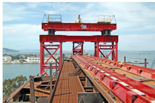
Figure 2. Construction work takes place at a height of 50 m (Syrinx Industrial Electronics, www.syrinx.nl )
