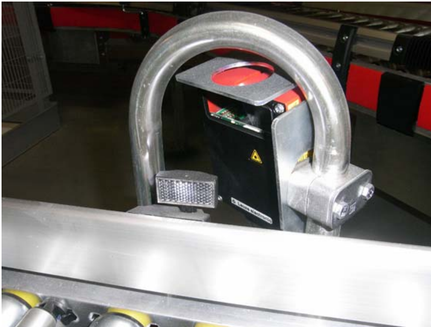
Figure 3. High-quality sensors are an important criterion for the profitability and availability of mechanical logistics systems – Leuze electronic supplied all the sensor components for the Future distribution center in Leipzig.
